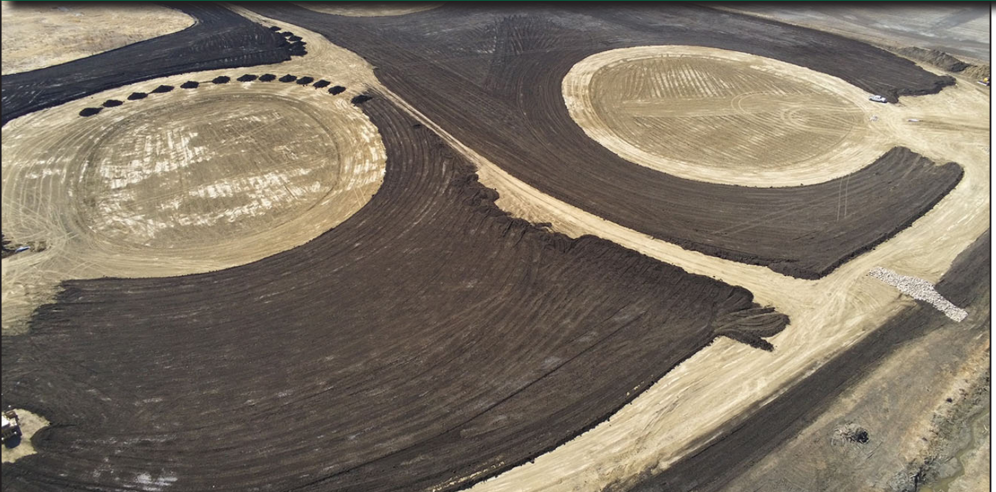
Town of Westlock Storm Water Infrastructure Project MPE Engineering Ltd. and Pidherney's Inc.
